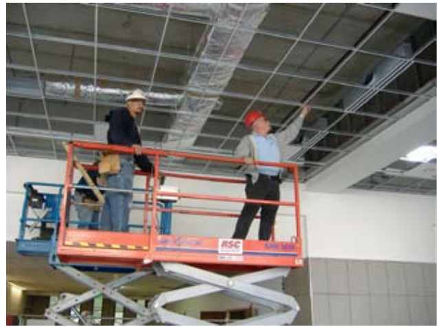
(Above) Workers from Belonger Corporation attend to tasks during construction on the Milwaukee Intermodal Station.
